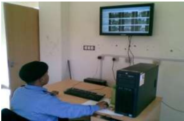
Control Room for CCTV
